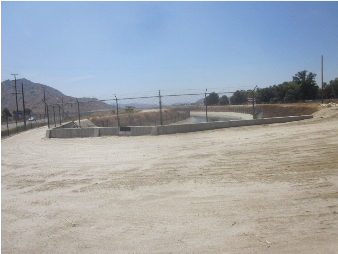
Overview of San Diego Aqueduct System, San Diego Canal P-33-015734 (view to south)
