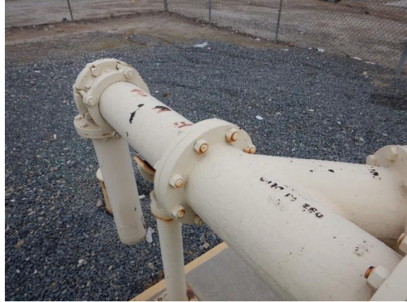
Photo 4.34-4 – Rust staining at flanges/bolts where coating has thinned (typical)
