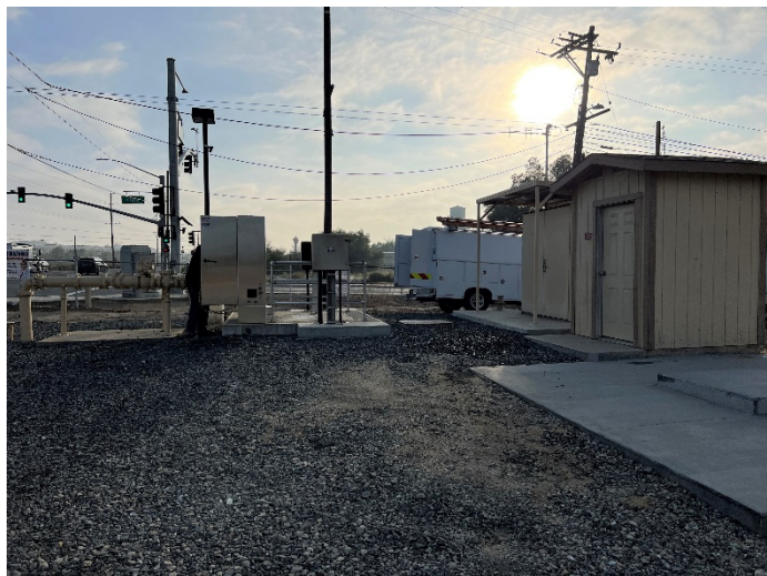
Clark Street Lift Station
