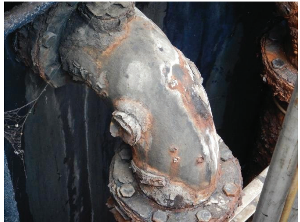
Photo 4.34-10 – Coating failure and corrosion on discharge piping (closeup)
