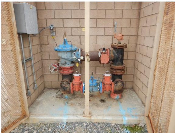
Photo 4.34-5 – Mead Valley Regulated Zone Piping Assembly
