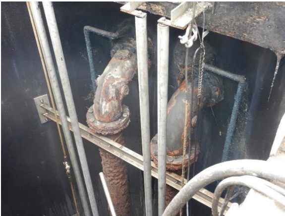
Photo 4.34-9 – Submersible pump discharge piping heavily corroded throughout
