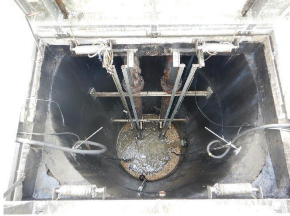
Photo 4.34-8 – Wet well, topside
