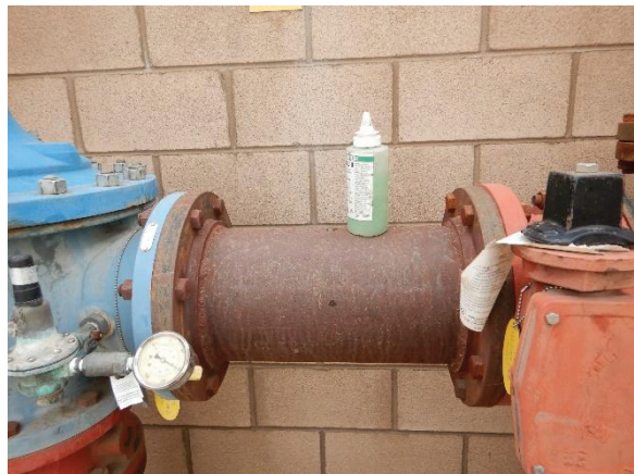
Photo 4.34-6 – Regulated Zone Piping Assembly UT-4 location
