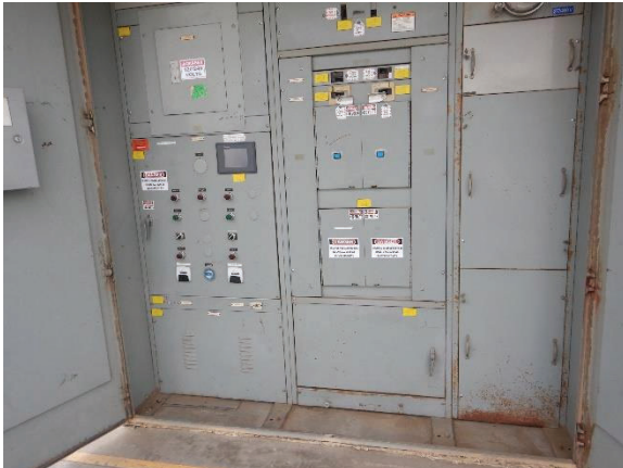
Photo 4.34-13 – Corrosion throughout electrical panels
