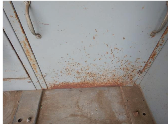
Photo 4.34-14 – Corrosion throughout electrical panels (typical)
