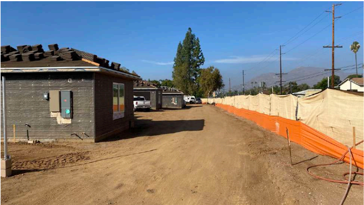
Photograph 6. MW-05a, eastern extent of project site facing west, entire location was under construction upon arrival.
