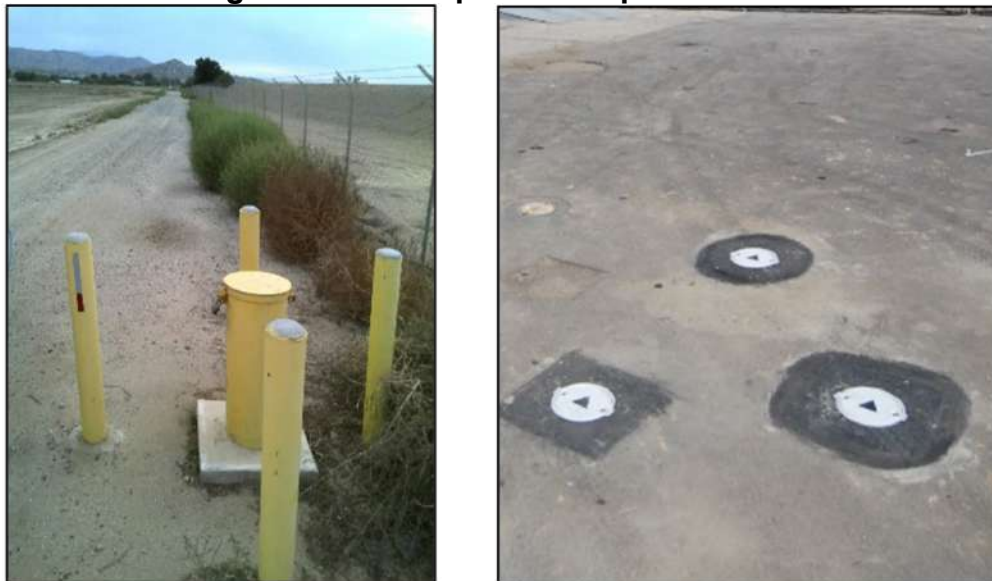
Example of aboveground wellheads (left) and flush-mounted well heads (right).
