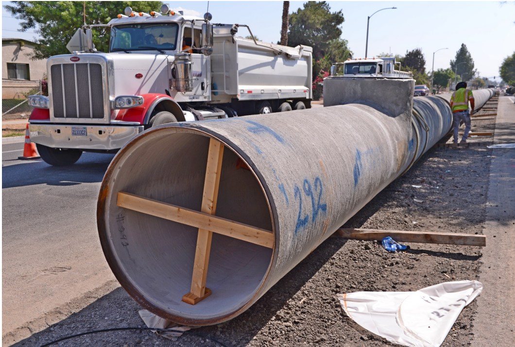
Phase 1 Feeder Construction: 42-inch CML&C pipe staged along Alessandro Blvd, looking East
