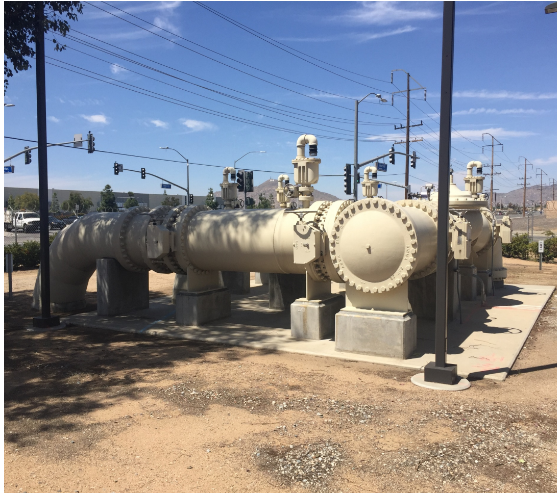
Typical turnout facility
