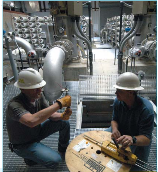
Construction of the Perris Desalter Phase 1 was helped by a $15 million grant from proposition 13 funds.
