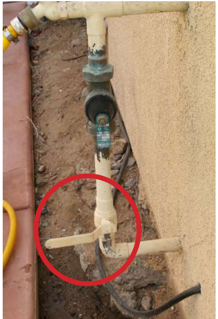
Water at house is "off"
