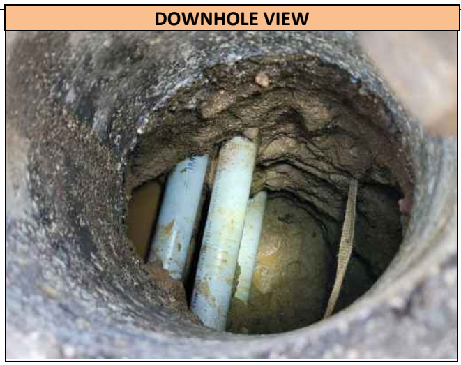
A downhole view of the utilities found in Pothole 30 and their orientation at the pothole location: 3.0 inch PVC Electric utility at the depth of 34.0 inches T/P and runs in a N/S direction; 1.0 inch wide PVC Package housing Telecom utilities found at the depth of 16.0 inches T/Pkg running in a N/S direction. Utilities were found directly on markout.
