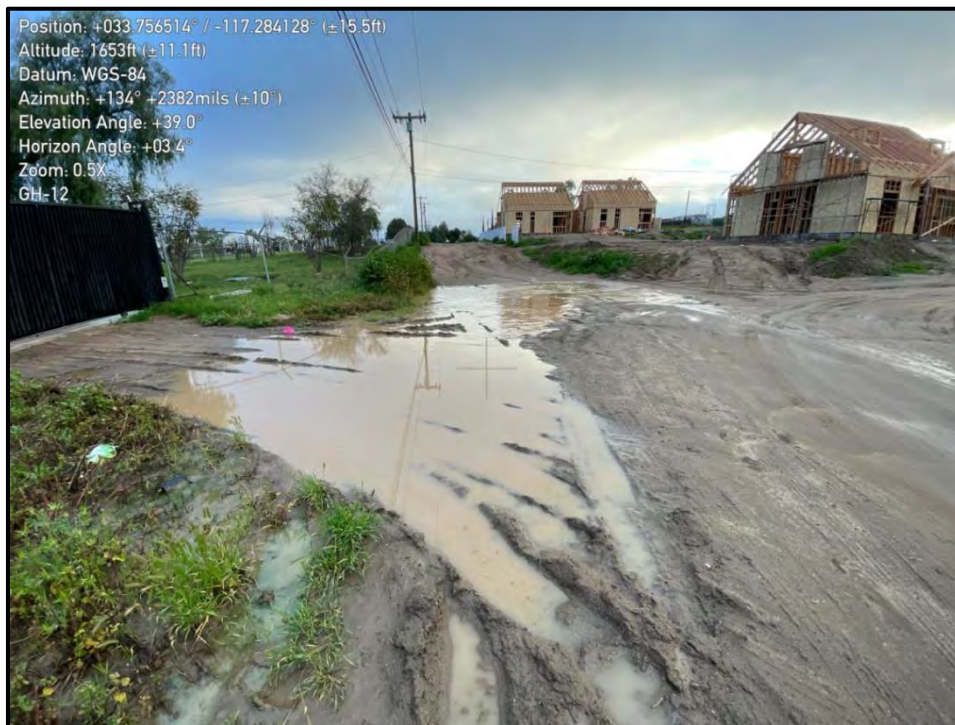
Photo 4: Large ponding at feature "GH-12" in the northern portion of the project.
