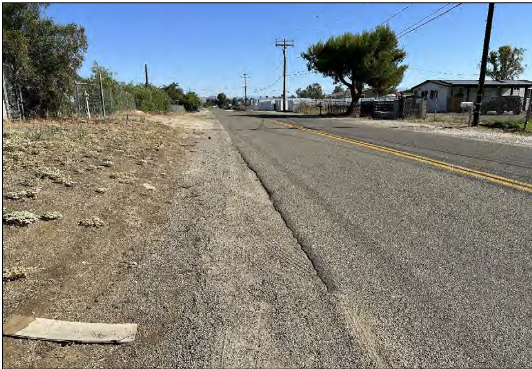
Figure 4 Carroll Street right-of-way from its intersection with Pinewood Street in Mead Valley portion; facing north.
