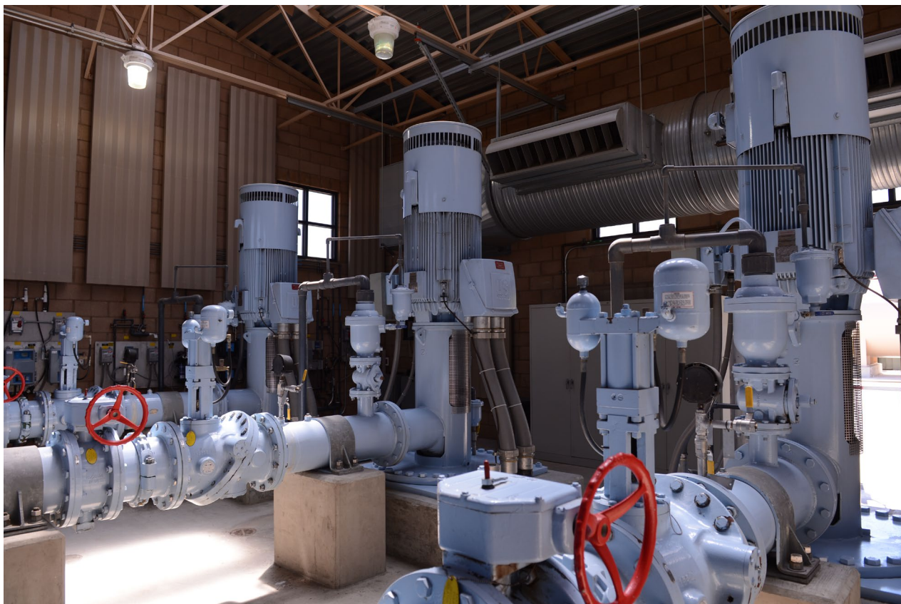
Pumps at Hemet Water Filtrations Plant
